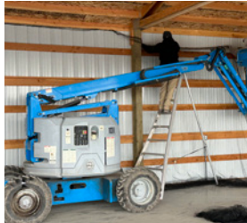
Pro Ag Services installing bird netting in the new Stuart Gallion Building
