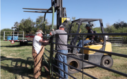
Alan Geho & Dave Sheuffele putting together the round pen. George on forklift providing the 'lift'
