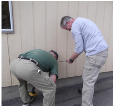
Bill McLaughlin & Don Evans pulling the cable through the office wall to install the Starlink satellite antenna
