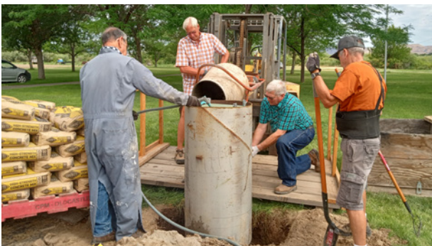
Day 1 of concrete pour at base of post for John Deere sign. Mike Haider, John Kobli, Vaughn Warren, Nick Schultz
