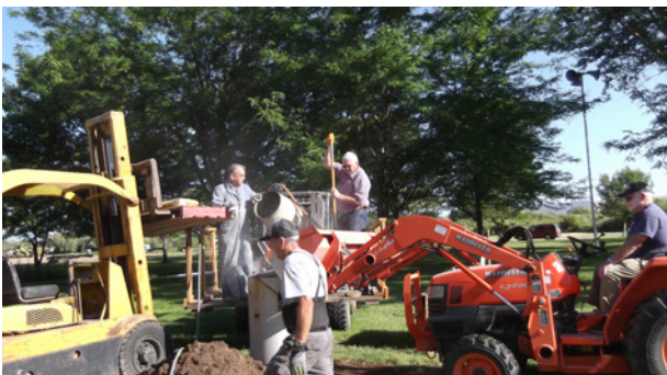
Day 2 adding gravel with the concrete inside sign post. Mike, Nick, Vaughn, Bill McLaughlin
