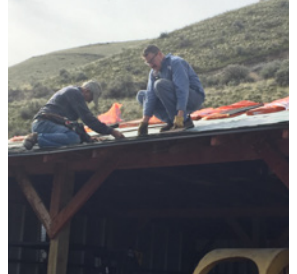
Bill Driskill & Jim Kabrich replacing the roof on the forklift garage in April 2022, five months before Bill passed at 92
