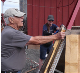
Harvey Cleem and Tami using chalk-line to mark a straight line at top of Merry-Go-Round base
